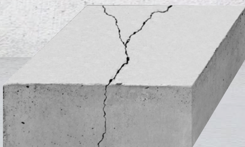
Random cracking is amongst the most costly and aggravating problems facing concrete contractors.
